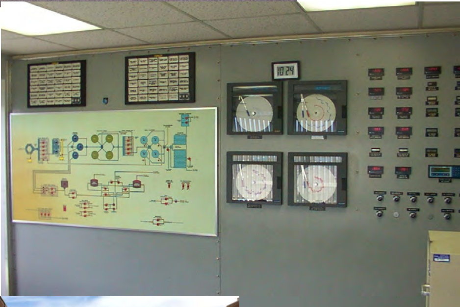
North Treatment Plant Operation Control Panel
